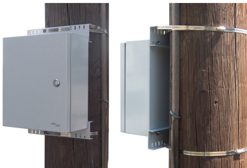
TerraWave Flex-Line Universal Steel Enclosure Mounted to Large Telephone Pole
