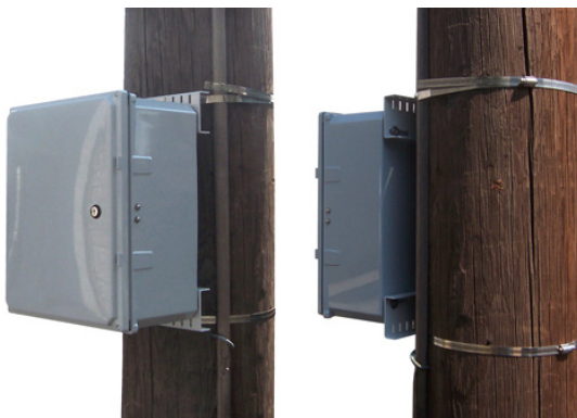
TerraWave Polycarbonate Enclosure Mounted to Large Telephone Pole
